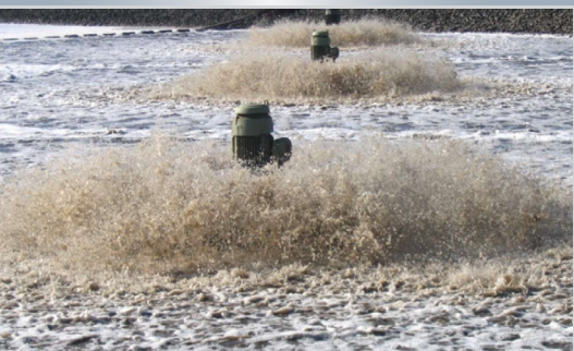
➔ Reduction of Aerator requirement Saving 70-80% Electricity
